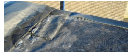
Defects require remedying
